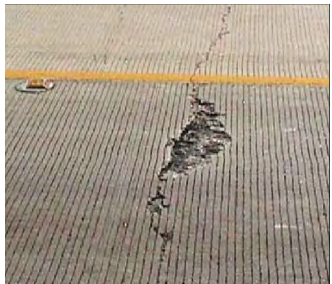
Figure 9. Spalling along transverse crack in a CRCP.
