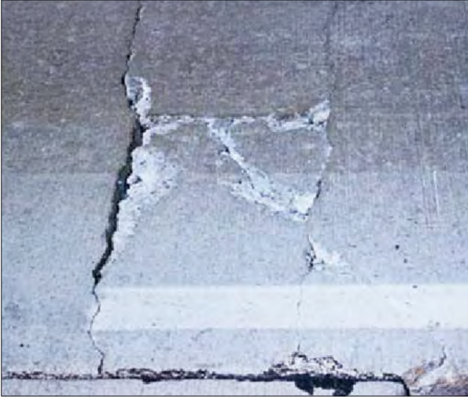
Figure 7. A typical CRCP punchout distress.
