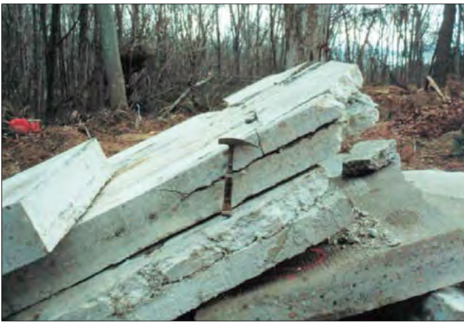
Figure 10. Horizontal cracking plane in CRCP.
